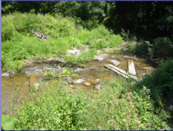
Figure 11. Looking north at partial breach section
