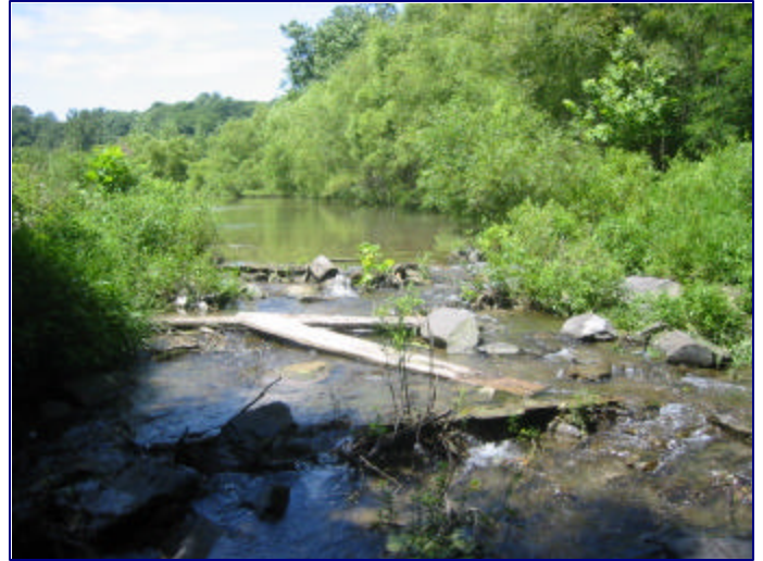
Figure 12. Looking north at partial breach section
